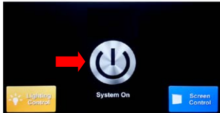
(Photo 1) Touch Panel and System On
